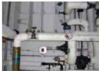
Asbestos insulation on pipes
