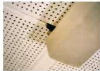
Asbestos insulating board ceiling tiles
