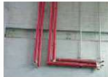
Asbestos lagging on pipes
