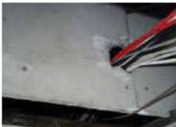
Asbestos insulating board panels
